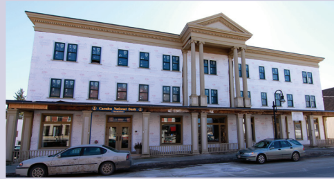
Knox Hotel Apartments under renovation in Thomaston. When completed it will provide 29 affordable units for seniors.
