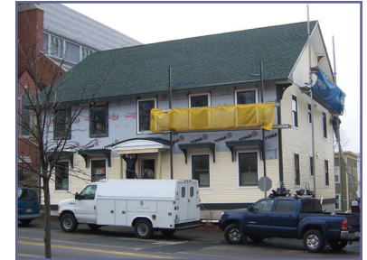
My Sister's Place under construction in Biddeford. It provided jobs while being rehabilitated, and now provides 4 units of housing for people who were homeless.
