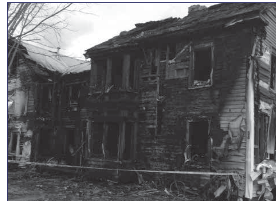
A two-story apartment building in Norway owned by Peter Marcinuk was destroyed by fire in October. Tenants got out safely.
